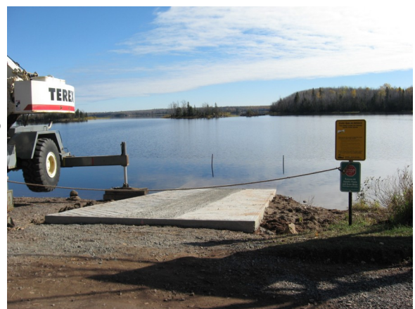
... to a poured concrete landing that will provide a safe launch facility for boaters while protecting the shoreline
