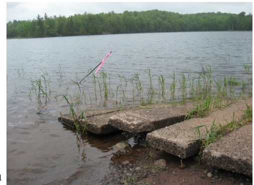
From this, a safety hazard for boaters and an erosion problem
